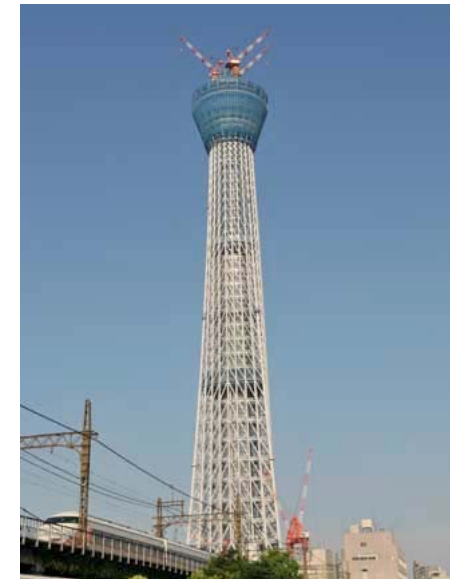
A recent picture of the Sky Tree under construction, at a height of 398 meters.
